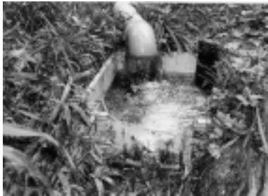
A weir installed in the Hyakumakidani stream.
